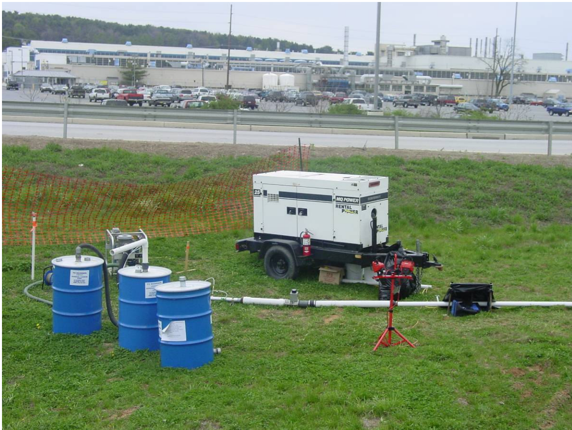
Photograph 4 – 50 KW generator and light stand.
