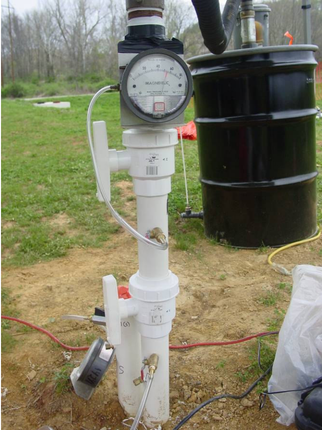
Photograph 8 – SVE extraction well sampling ports and vacuum flow measurement.
