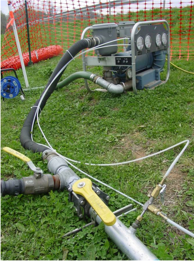
Photograph 7 – SVE connections to blower and flow measurement port.
