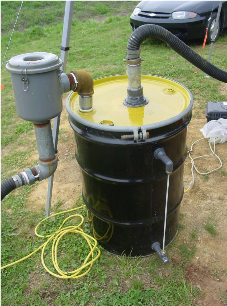
Photograph 5 – Knockout drum and connections.
