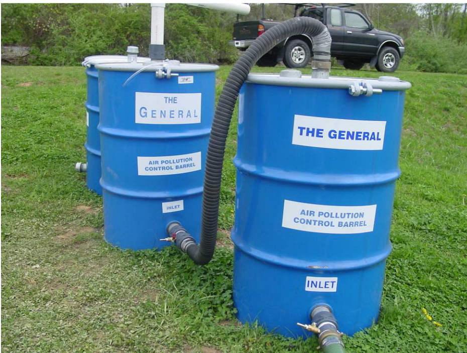
Photograph 6 – Granular activated carbon drums and connections
